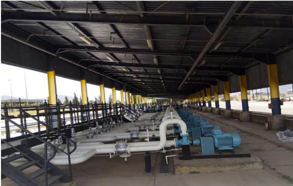
Figure I-3: Station de pompage.[4]
