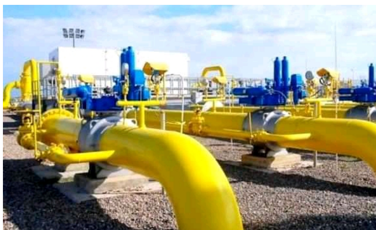
FIGURE 2.2 – Station de distribution du gaz
