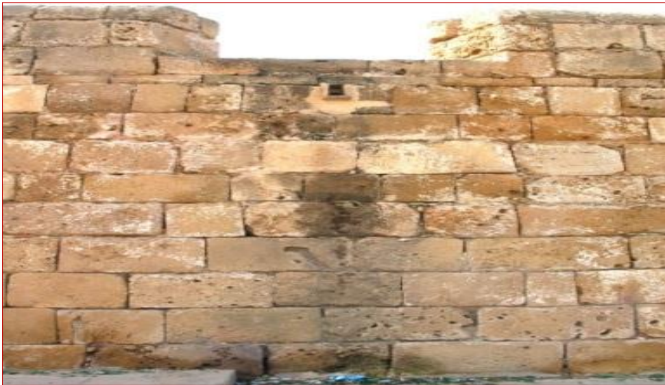
Figure 124: Apparition des noircissures
