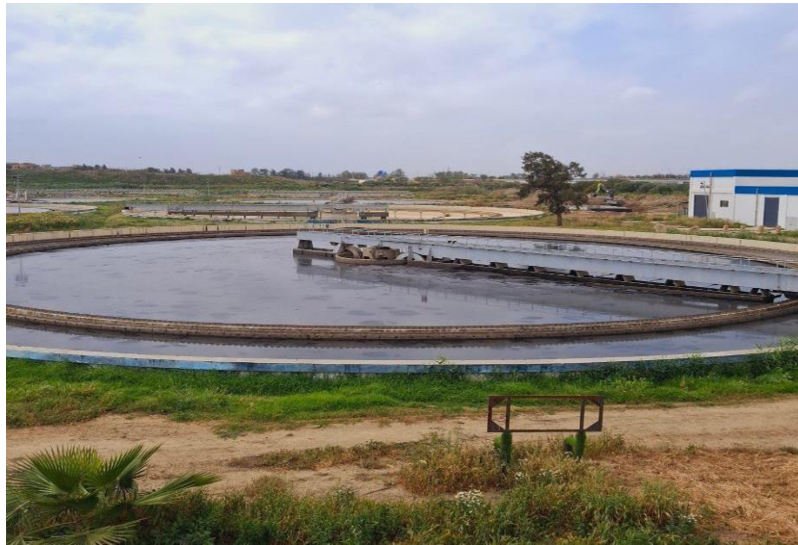
Figure 9 : Clarificateur (photo originale)
