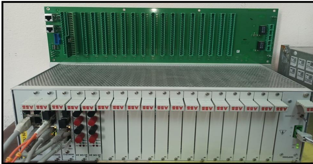
Figure 2. 7: RTU 560 ABB de la SONELGAZ BLIDA .
