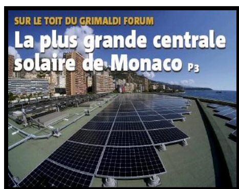
Figure 27: la plus grande centrale solaire de Monaco Source : https://www.pressreader.com/monaco/monaco-matin/20190921/283029761324588
