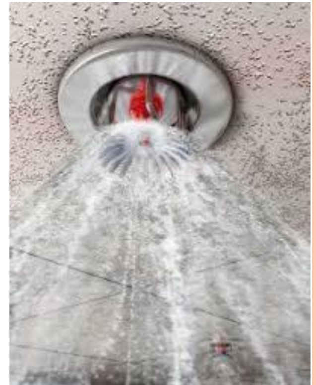
Fig, Spinklers ; https://dir.indiamart. com/indore/fire- sprinkler- system.html
