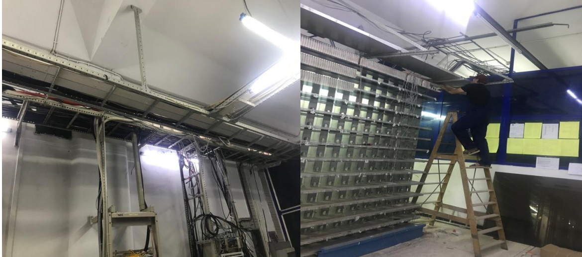
Figure II. 27: Le chemin de câble
