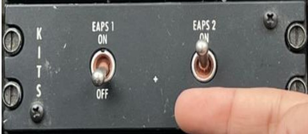
Figure 4.3: EAPS control switch
