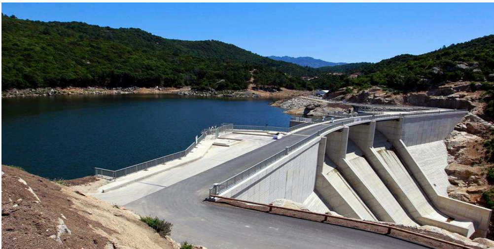
Figure (I.11) : Barrages Hydraulique [14]
