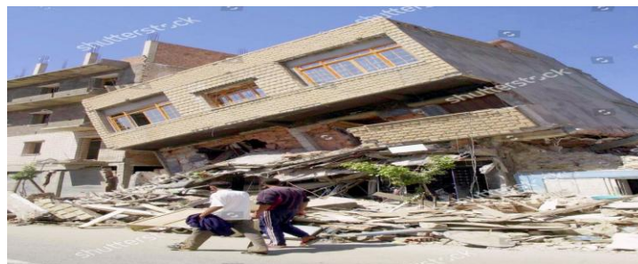
Figure1.5.1 Damaged building (earthquake Boumerdes2003)
