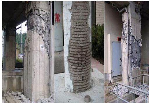
Figure 1.6.1 Column failures due to compression
