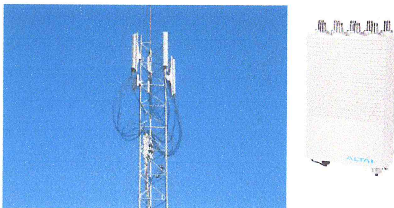
Figure 2.11 : La station de Base A8 [13]
