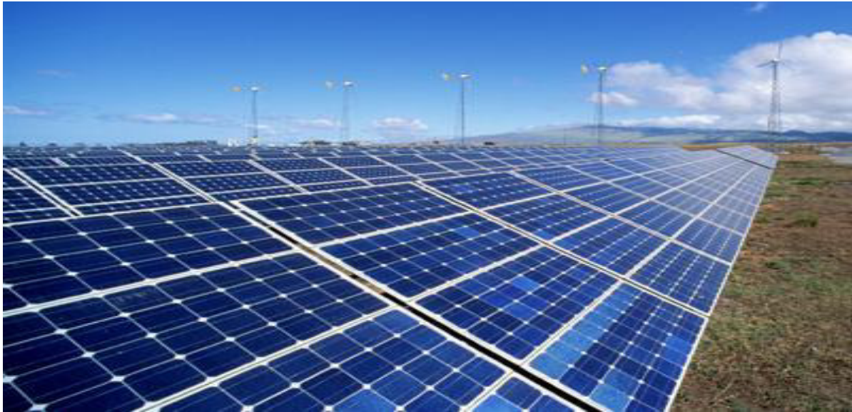
Figure I.8 : La Solaire photovoltaïque [6]
