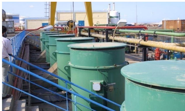
Figure I.13 Station de pompage
