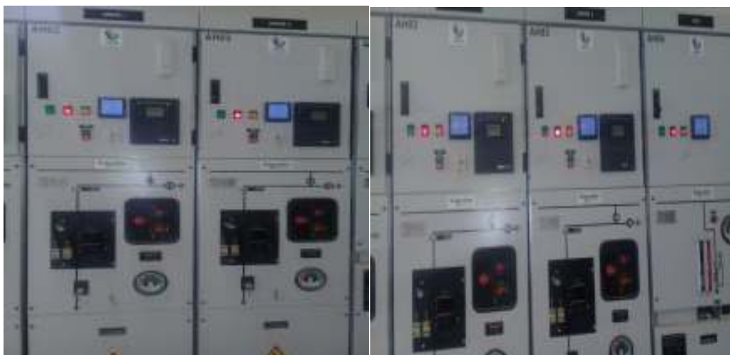
Figure II.9 :L'armoire de central
