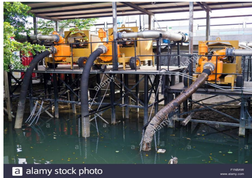
Station de pompage Source : https://www.istockphoto.com/
