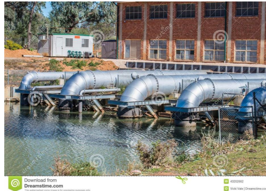
Station de pompage Source : https://www.istockphoto.com/
