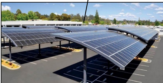
Figure 130 Solar panel parking roof /source: indiamart.com
