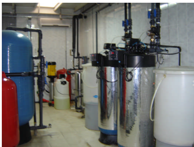
Figure 30: Salle de filtration ©ZM
