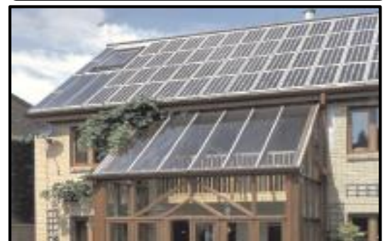
Fig28.1: panneaux photovoltaïque Source: www.google image.com
