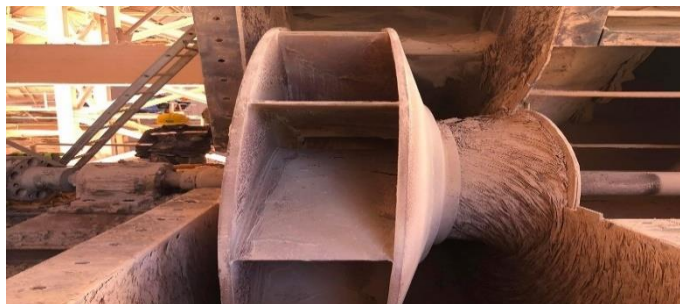
Figure 3.24 Colmatage de la turbine.
