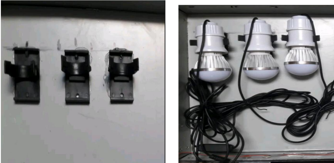
Figure (III-14) : Installation de lampes LED.
