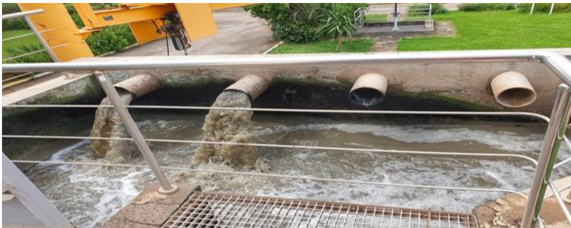
Figure 2.5: poste de relevage.
