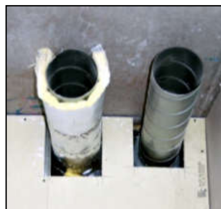
Figure 27:tuyau de ventilation double flux
