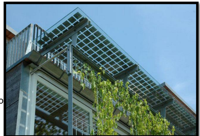
Sunshading solar panels
