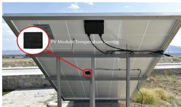
Figure 2.11: Back-of PV panel Temperature sensor [56].
