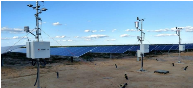
Figure 2.9: PV weather stations installed in a PV ground [51].
