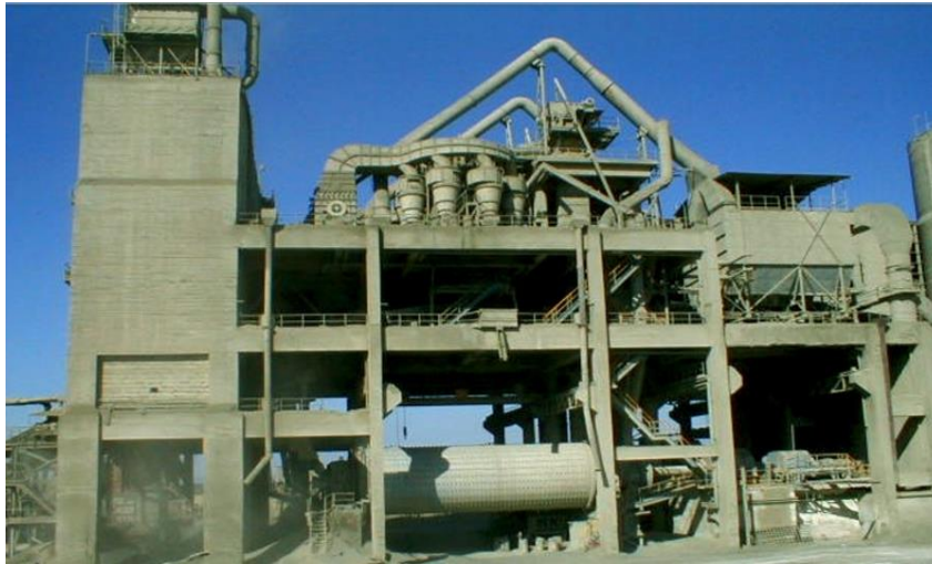
Figure 1.2 : Atelier broyage ciment
