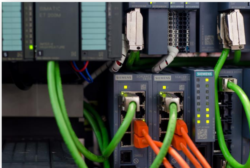
Figure 18 Automate programmable PLC siemens
