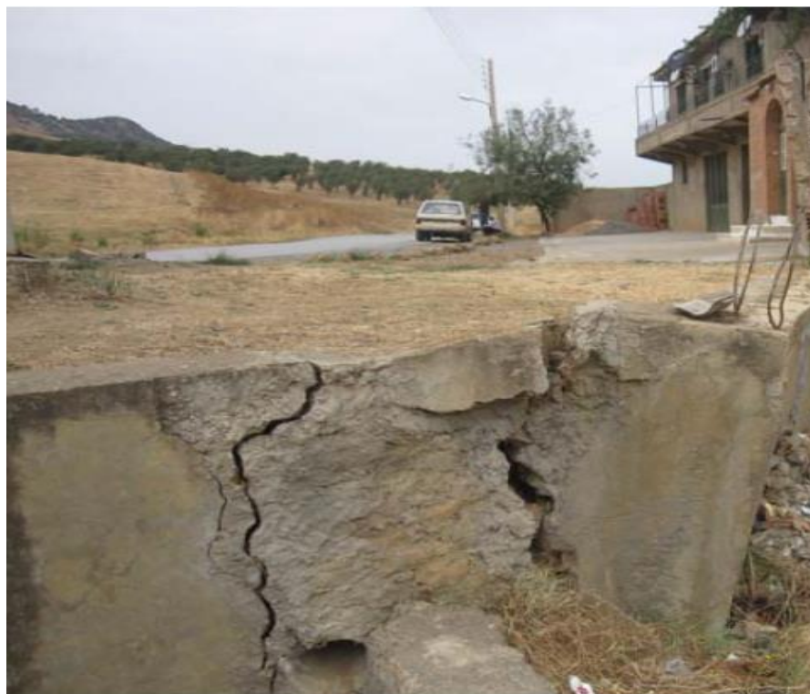
Figure II.6 : Rupture du muret.
