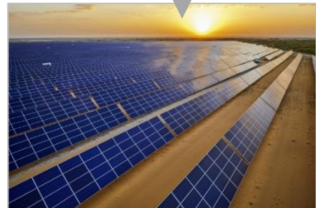
Figure ICVI.70: panneaux solaires Source : https://cutt.ly/iwulvqCj
