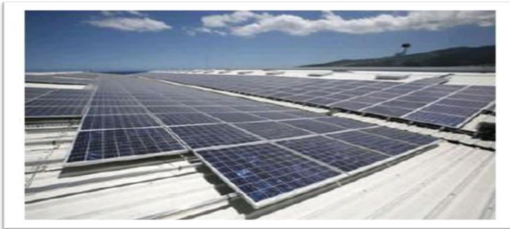
Figure I-4 Panneaux Solaires Photovoltaïque
