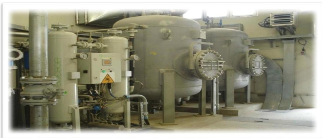
Figure 3.13: Station d'air comprimé .
