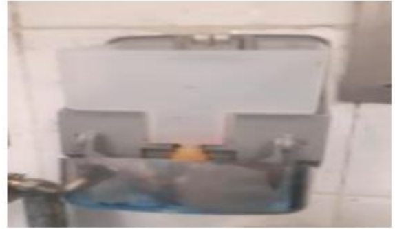
Figure 23 : Absence de lave main coté Alcip 10/100. (Photographie originale)
