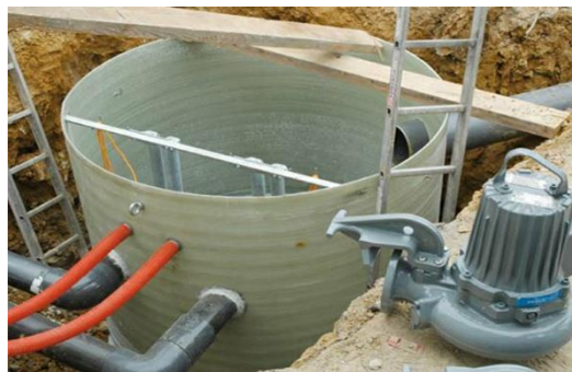
Figure IV 31. Station de relevage
