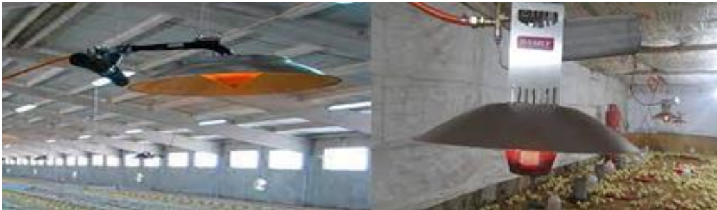
Figure 17: Les chauffages radiant(38).
