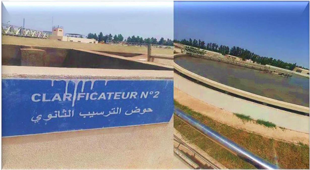
Figure 1. 5 : Clarification de STEP de Beni Merad (Photo original 2024).
