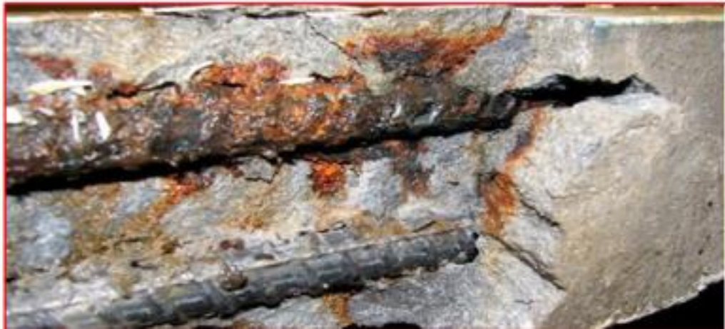
Figure I.2 : Corrosion Des Aciers [1]
