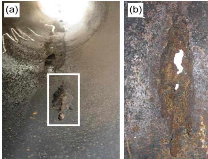
Figure 2-5: (a) corrosion, (b) erosion [15].
