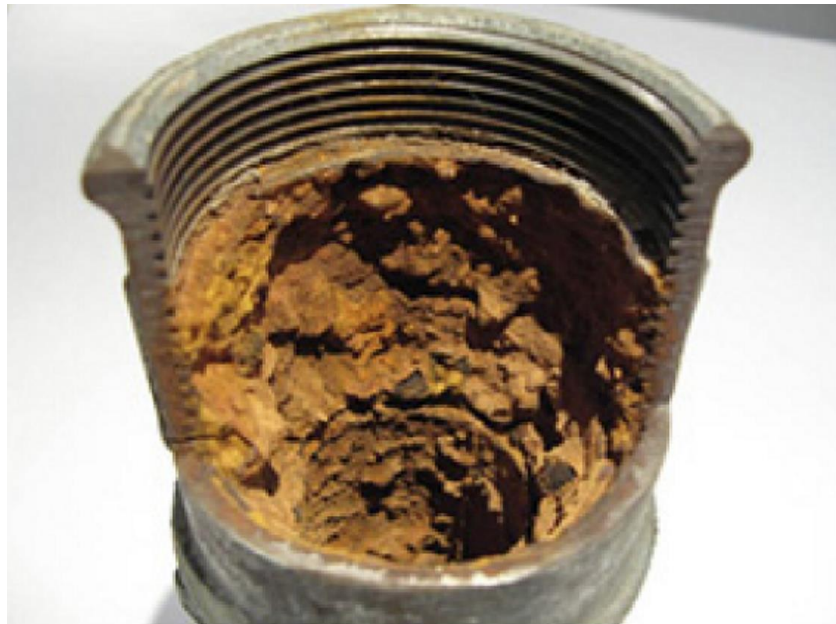
Figure 2-6: Formation of scale in the pipe.
