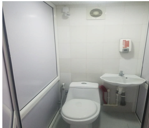
Figure 11 : Laves mains /Toilettes.
