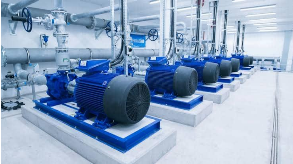
Figure 1.2. Station de pompage.
