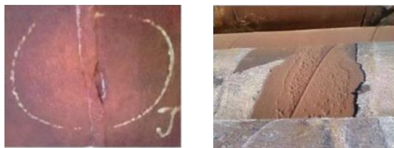
Figure I.3: Corrosion des pipelines.
