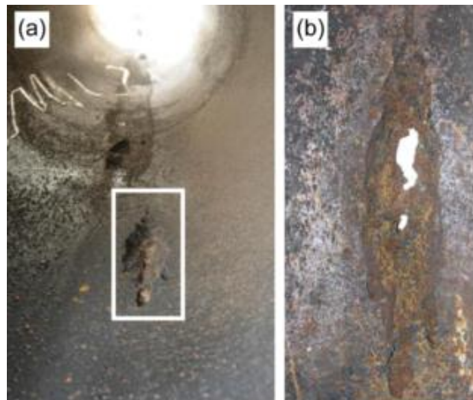
Figure II.5: The location internal corrosion on subsea pipe elbow [9].
