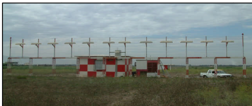
Figure III. 15. Station LLZ à Alger.
