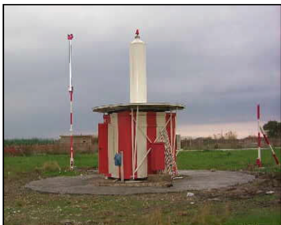
Figure III.3. Station CVOR à Alger
