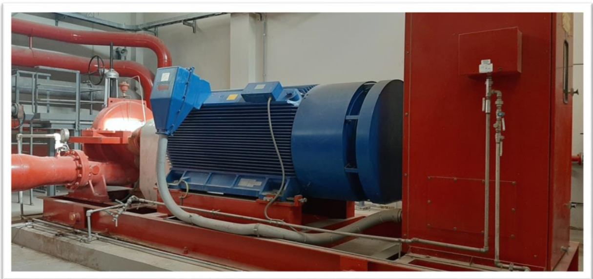
Figure 2.3 moto pompe principale 1
