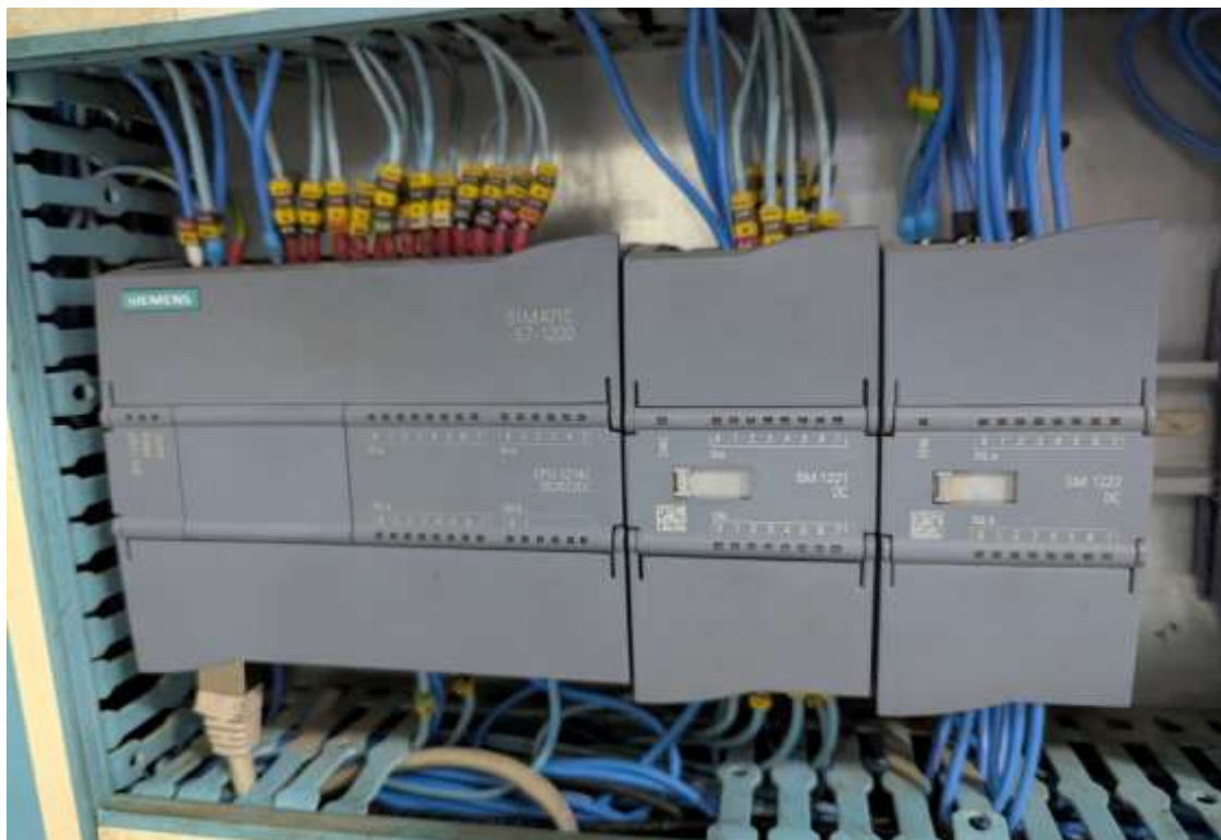
Figure 2. 5: l'automate Siemens S7-1200 [15]
