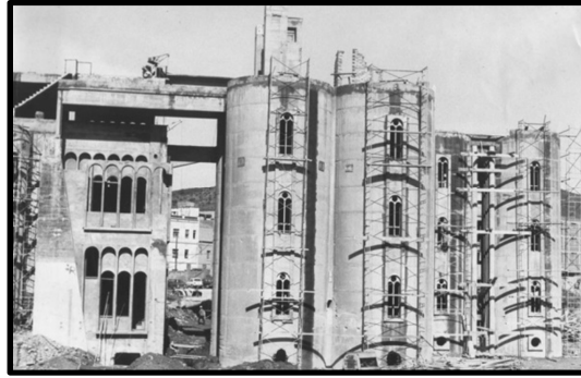
Figure 100 : vue de la cimenterie en plein travaux, source: Ytazer , a former cement factory is now the workspace and residence of Ricardo Bofill
