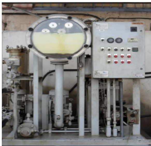
Figure II.2 : Station de déshydratation
