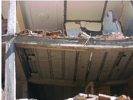
Figure 4. Damage of beams in flexure
