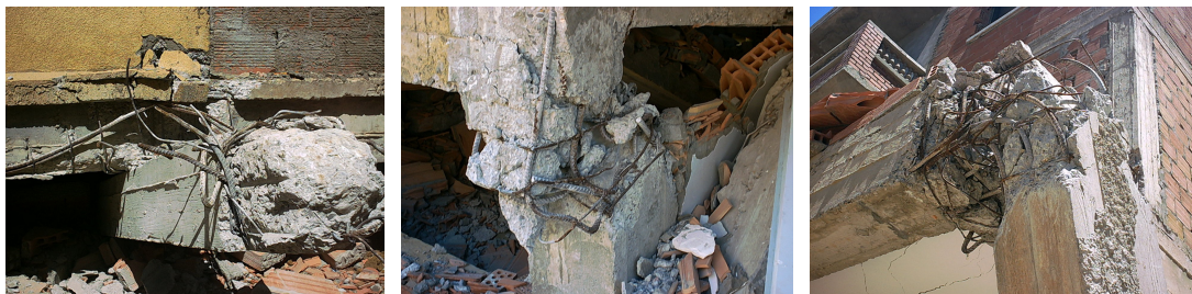
Figure 3. Typical local damage of columns
