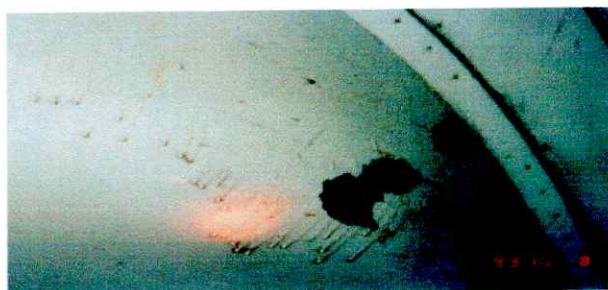
Figure B4 - Paint Peeling
