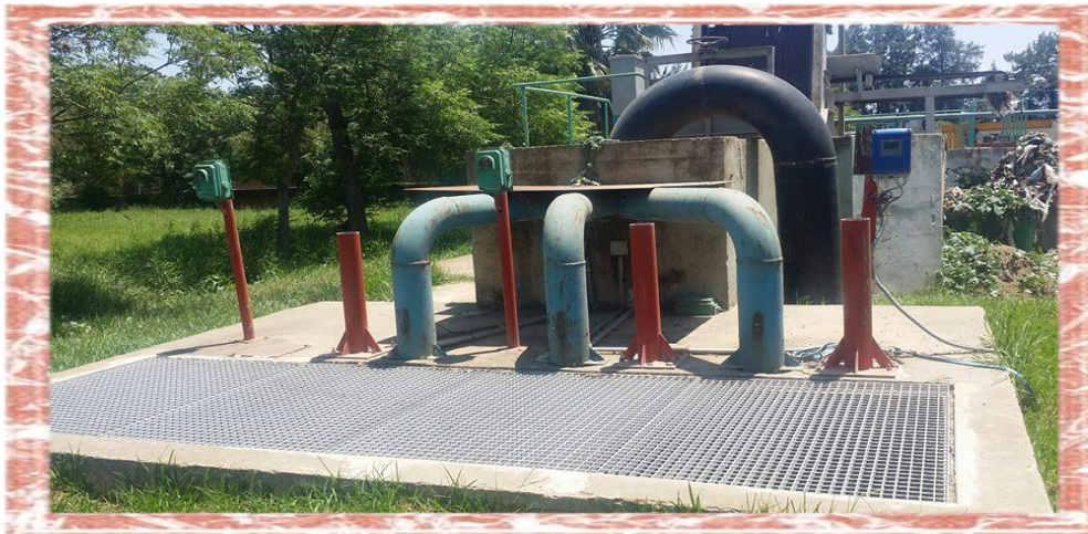
Figure N°03 : Station de relevage (photo originale)
