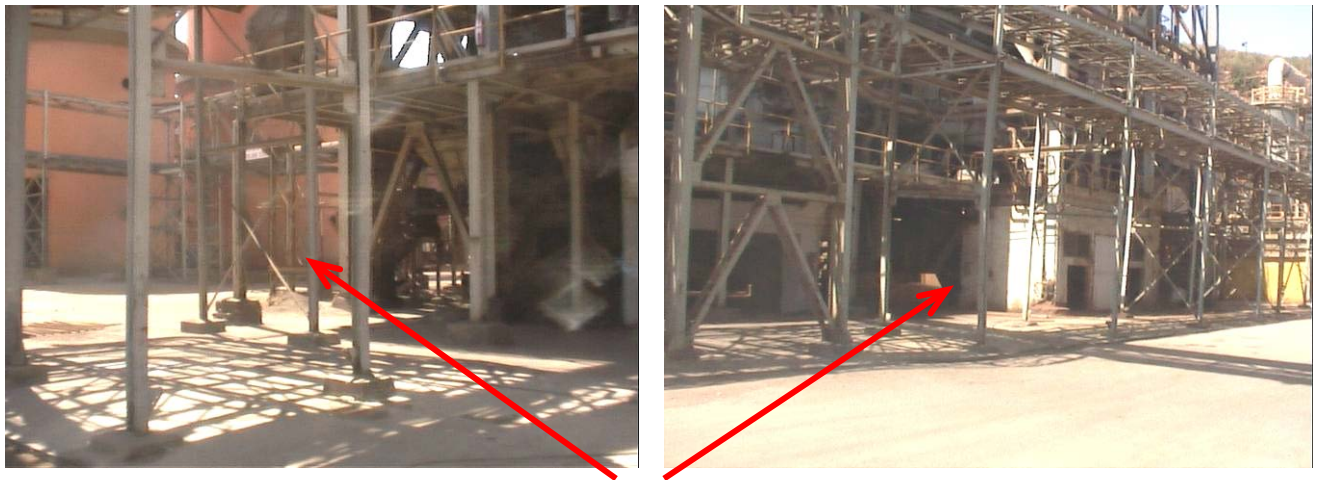
Figure 5.48 : Absence des contreventements.
